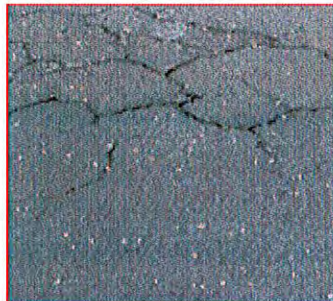
“Spider Web Cracking” caused by seal coating.
