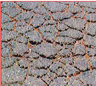
“Alligator Cracking” caused by seal coating.
